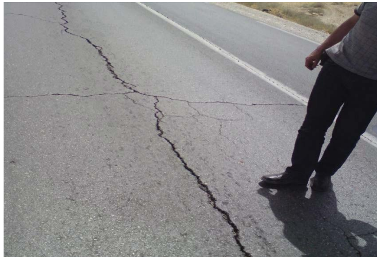
Figure 5. Cracking distress on pavement structure.
